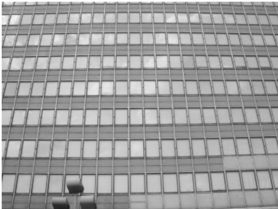
Plain facade, complex problems. (Photo: Hutter)
